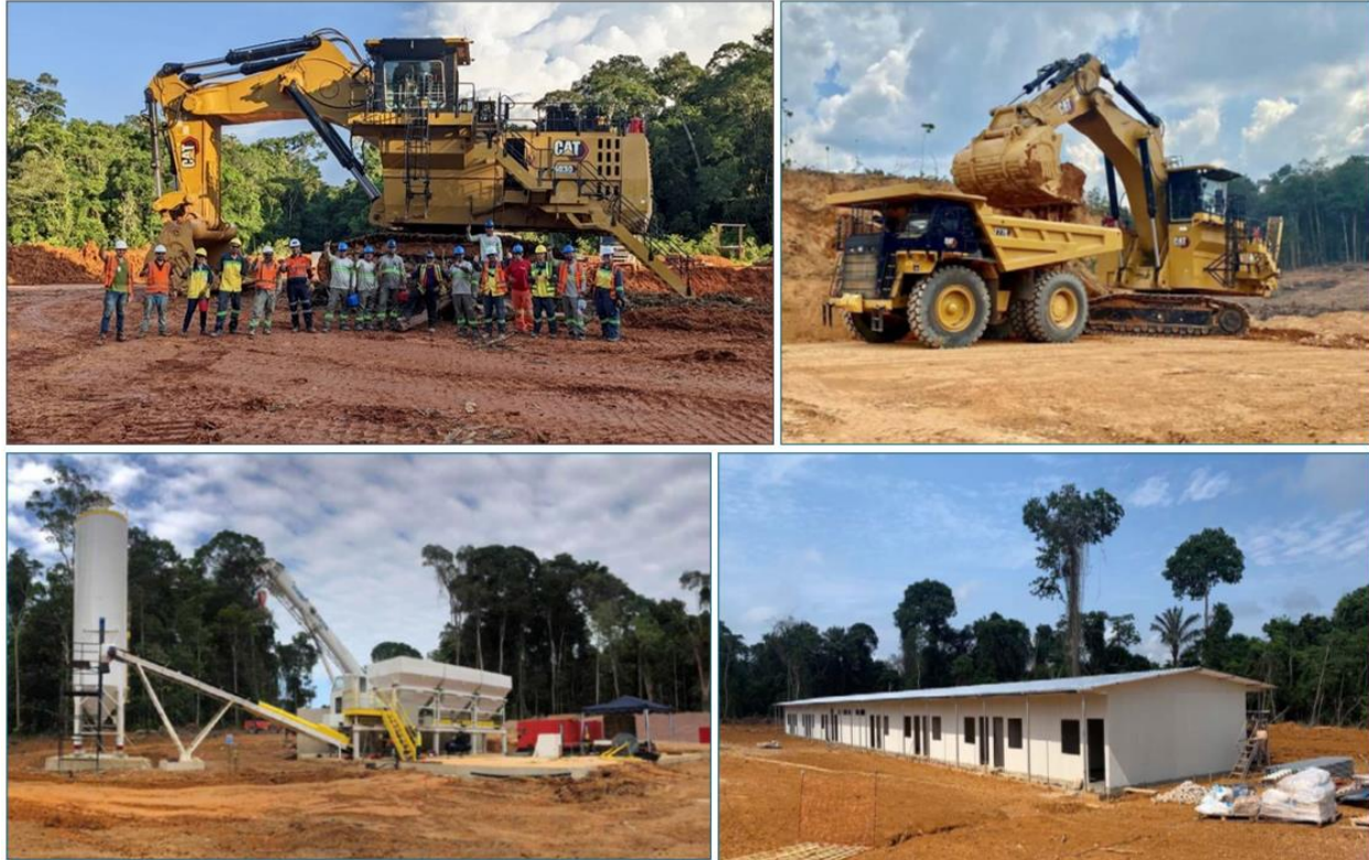
Figure 2: Tocantinzinho (A) personnel, (B) starter-pit mining, (C) concrete batch plant, and (B) camp
